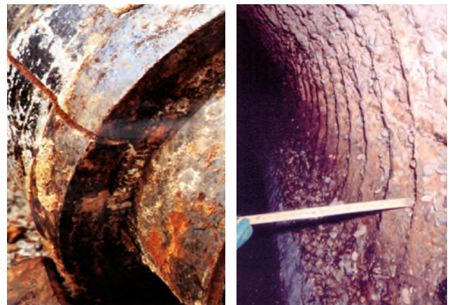
EXTERIOR AND INTERIOR CORROSION EFFECTS IN PIPING.
