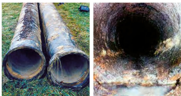
PIPING SUFFERING FROM ELECTRO-CHEMICAL CORROSION.
