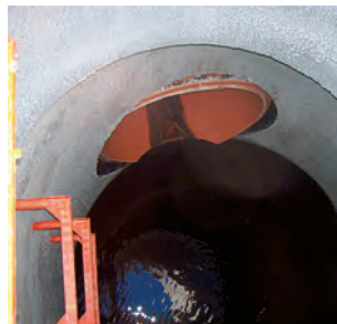
SEALING FAILURE IN CONCRETE MANHOLES.
