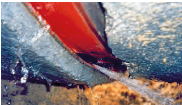
LEAKING AT A CONCRETE PIPELINE JOINT.
