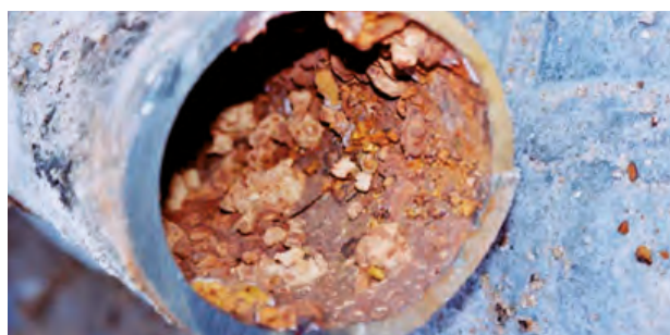
SEWAGE PIPING WITH MATERIAL DEPOSITS.
